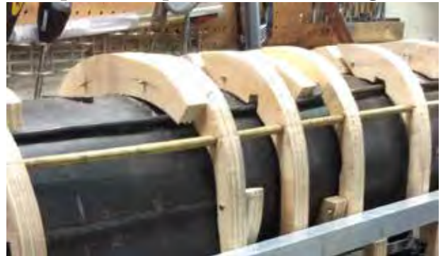
The new shroud forms were two piece with a pinned locking section used to hold them tighter onto the boiler shell. The throttle rod is inside the brass tube.
