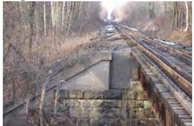
Chuck's picture of the Griggs Bridge showing the cement work above the stone block on the abutments.
